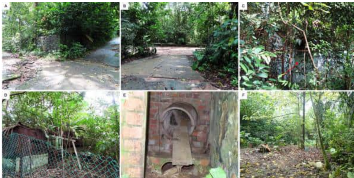
Figure 7-30 Infrastructure in Site B. (A–B) Concrete and sand pathways for horses; (C–D) Abandoned buildings within green chain-linked fences and with overgrown vegetation; (E) A Culvert; (F) Abandoned amenities.
